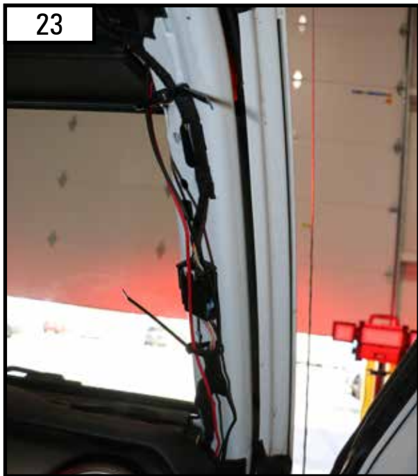
Run the wires down the A-pillar alongside the factory wiring. Use the zip ties provided.
